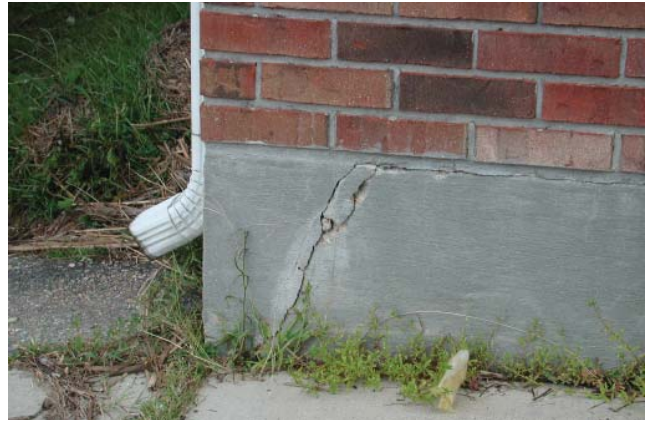
Photo 7 Crack at Foundation Due to Lack of Bond Break Between Brickwork and Concrete
