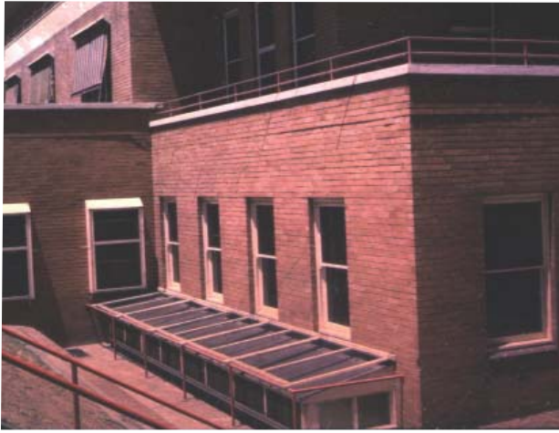
Photo 6 Movement of Parapet Away from Corner
