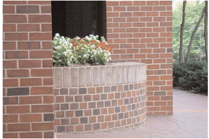
Figure 4 Brick Headers Used for a Small Radius Curve
